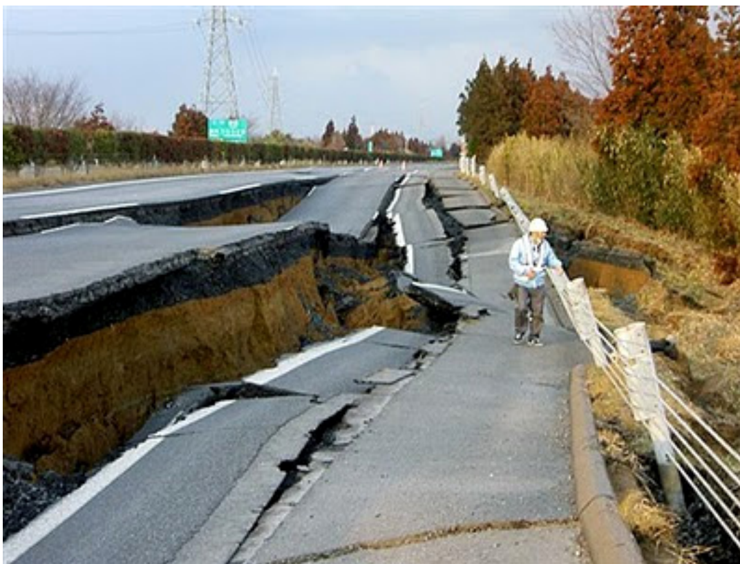
Slika 5. Avtocesta blizu kraja Mito v prefekturi Ibaraki po potresu (vir: http://noypistuff.blogspot.com/2011/03/japan-earthquake-2011-over-1000-people.html ) Figure 5. The Joban Motorway near Mito, Ibaraki Prefecture, after earthquake (source: http://noypistuff.blogspot.com/2011/03/japan-earthquake-2011-over-1000-people.html ).
