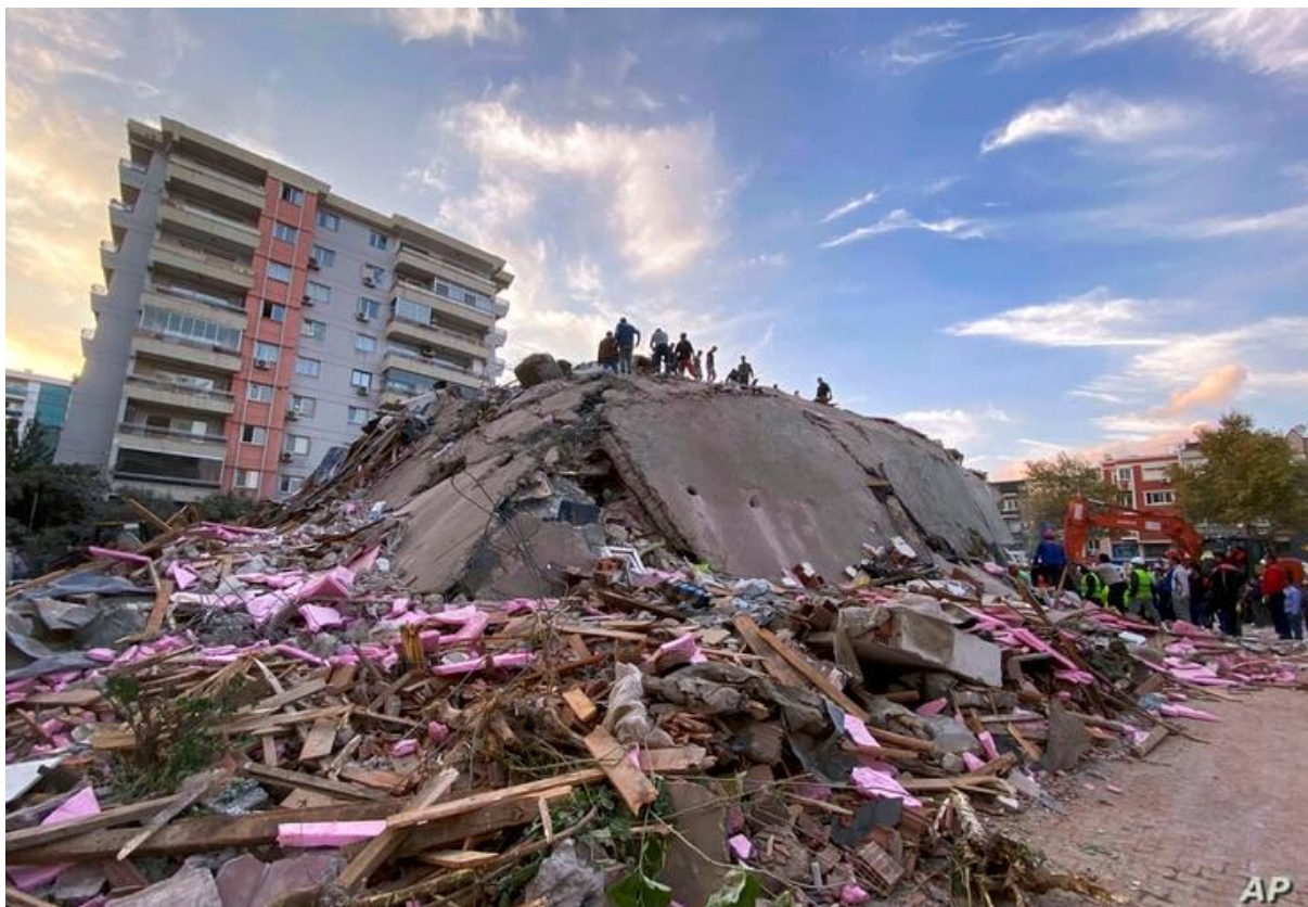
Slika 3. Popolnoma porušena zgradba v Izmirju, Turčija (vir: https://www.voanews.com/europe/powerful-quake-strikes-major-turkish-city-greek-islands ) Figure 3. A collapsed building in Izmir, Turkey (Source: https://www.voanews.com/europe/powerful-quake-strikes-major-turkish-city-greek-islands )
